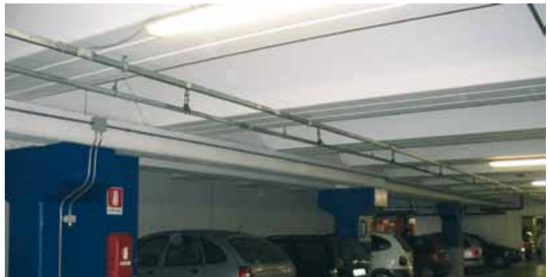
Canalis KBA supplying luminaires nearby sprinklers.
